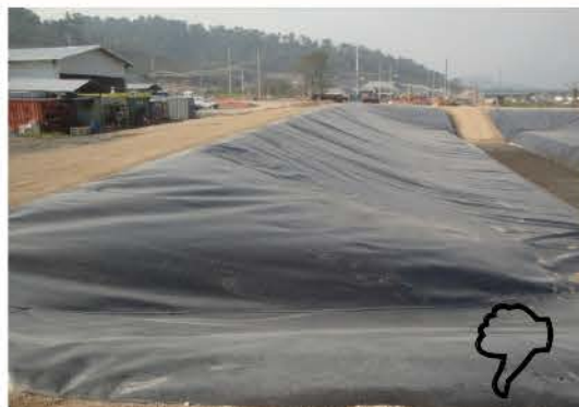
HDPE liner: wind uplift and wrinkles
